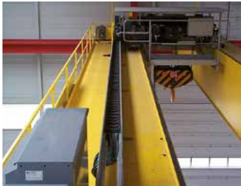
e-chainsystems® assembled on the crane girder
