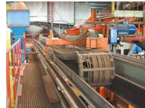
High loads as a result of brick dust
